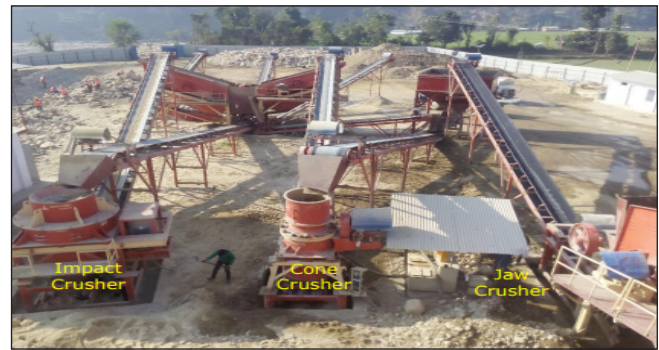
Figure 3. Crushing and Screening plant, BBDMP, Surkhet
