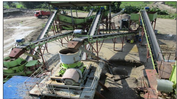
Figure 1. Crusher Plant, SMDMP, Sinduli (Source: Shrestha, 2022)
